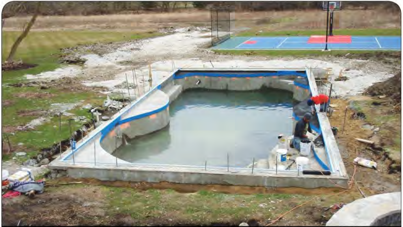
Accommodating the shape of the cover and the footings for cantilever requires a shell structure that contains far more concrete than an average pool and is built to the tightest possible tolerances. Executing these designs requires constant checking and rechecking of critical dimensions at each and every step of the process.
