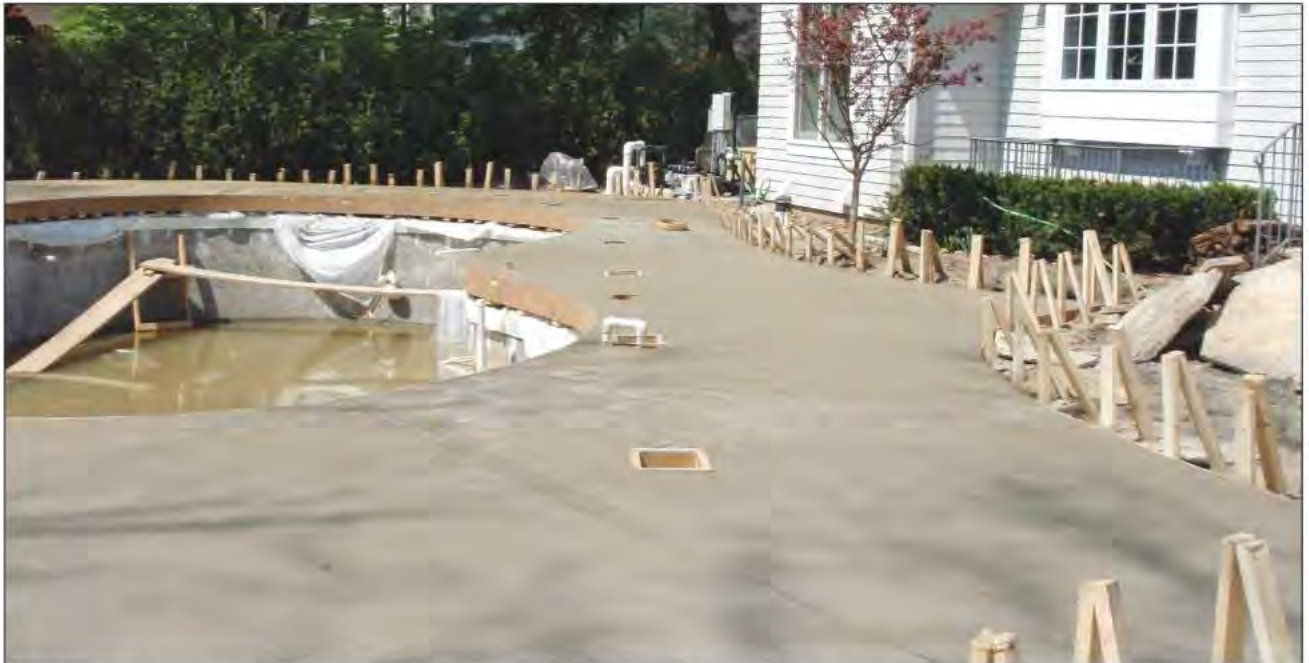
With the cantilever and surrounding deck cast in place, the cover's tracks are now completely concealed, save the openings we leave for future service.
