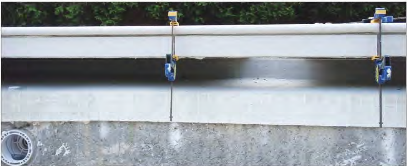
With all of the forms removed, the only remaining visual evidence of this advanced detail is the slot where the cover travels with the same ease as a more standard installation.
