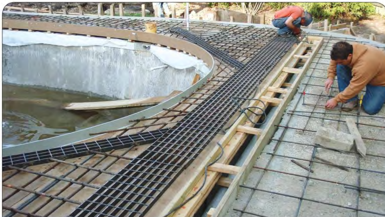
The cantilever structures are engineered and built using extensive reinforcing steel tied back to expanded footings. We often upsize footing dimensions and steel schedules beyond the engineers recommendation in order to add margins of structural strength.
